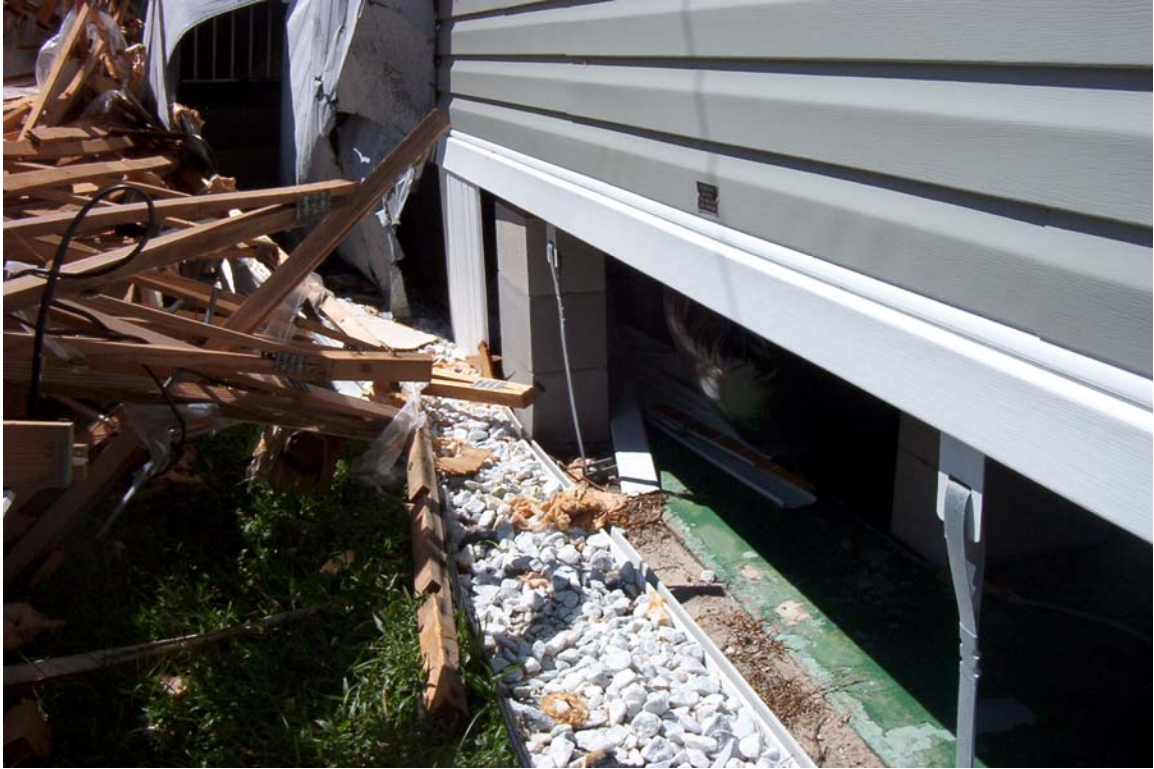
The home was installed by Mr. Diaz licensed mobile home installer IH0000295 Installer decal affixed to the home by Mr. Diaz. Decal # 195378
