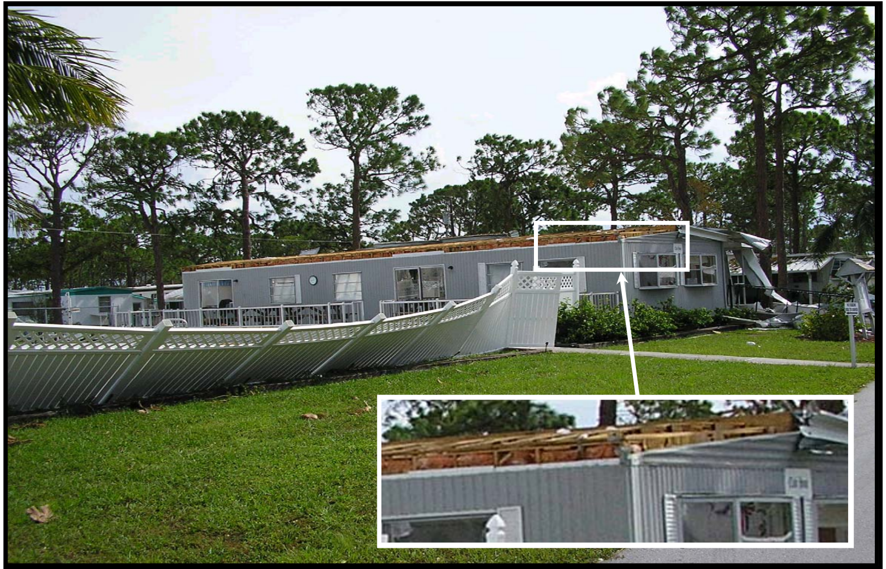
Shady Rest Mobile Home Park in Sebastian had this modified home being used as a clubhouse. It had an aluminum patio roof and it was attached to the clubhouse roof. When the patio roof was blown away it also took the clubhouse roof with it.
