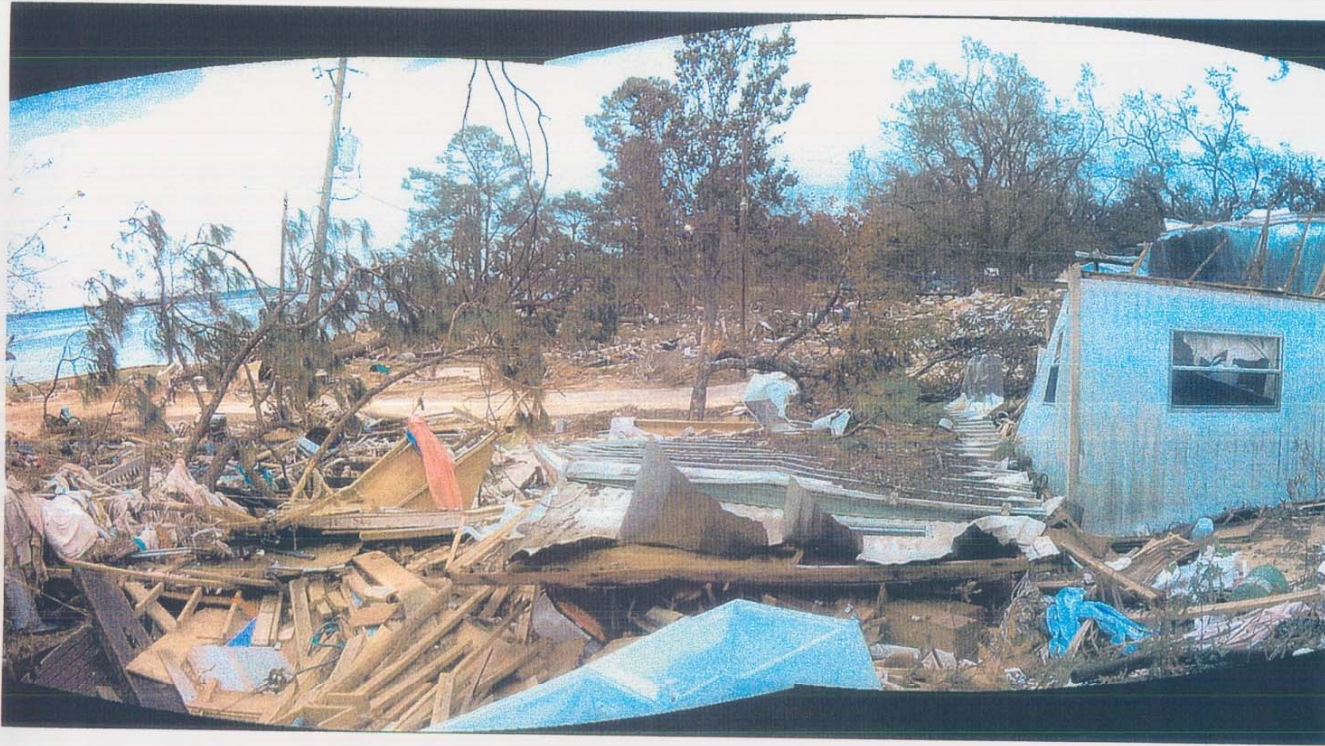
A panorama view of Bay Breeze MHP in Pace. 22 homes in this park and 6 were totally destroyed due to velocity/wave action. All homes were pre HUD and the many straps found on the frames had rusted away from the anchors.
