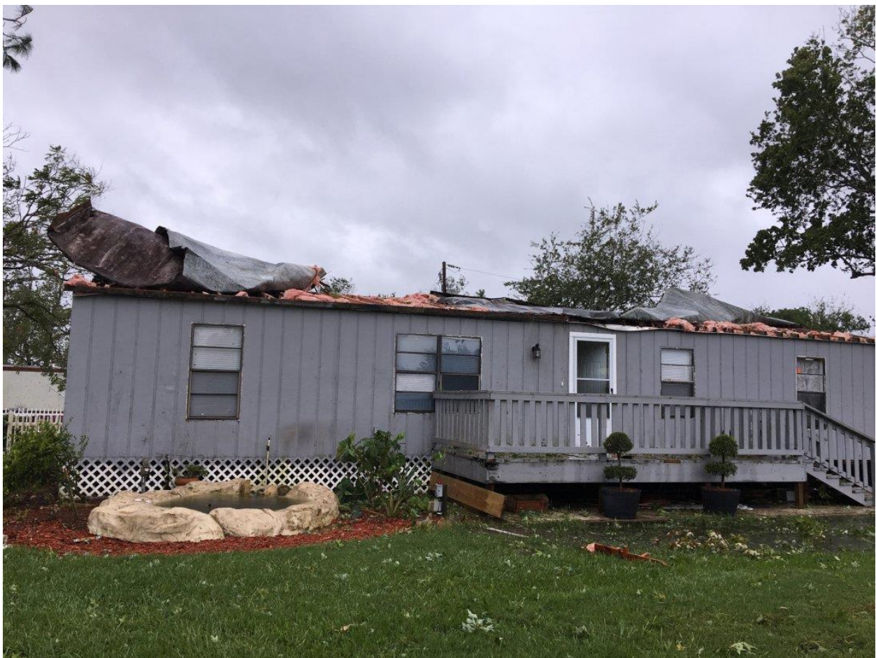
Mobile home damaged during Hurricane Matthew.
