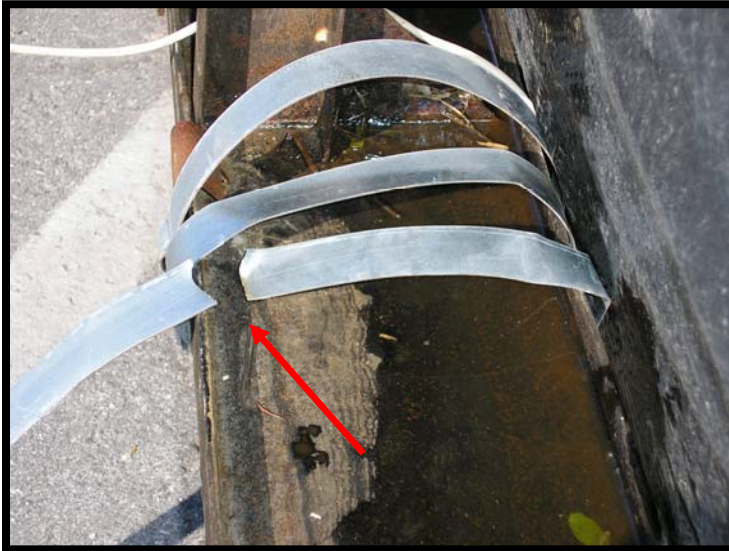
Straps wrap the I-beam causing breakage during tornadoes and high winds.
